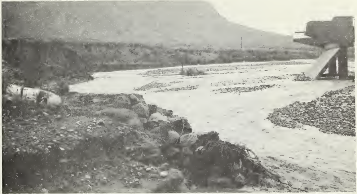
Bridge Damage Bridge on Highway 54 spanning Sulfur Draw The south abutment was washed out in August 1966.
